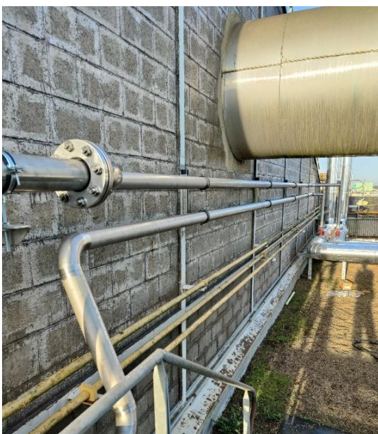
Industrial piping produced by Energy&+
